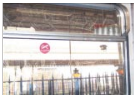
Glare and scratches on the window affect sign visibility
