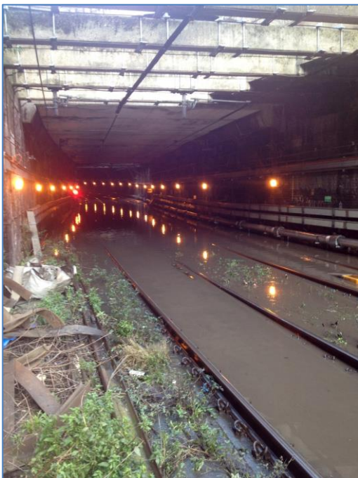
Floods at Clerkenwell Tunnel
