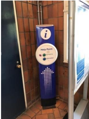
Figure 7- high visibility help point
