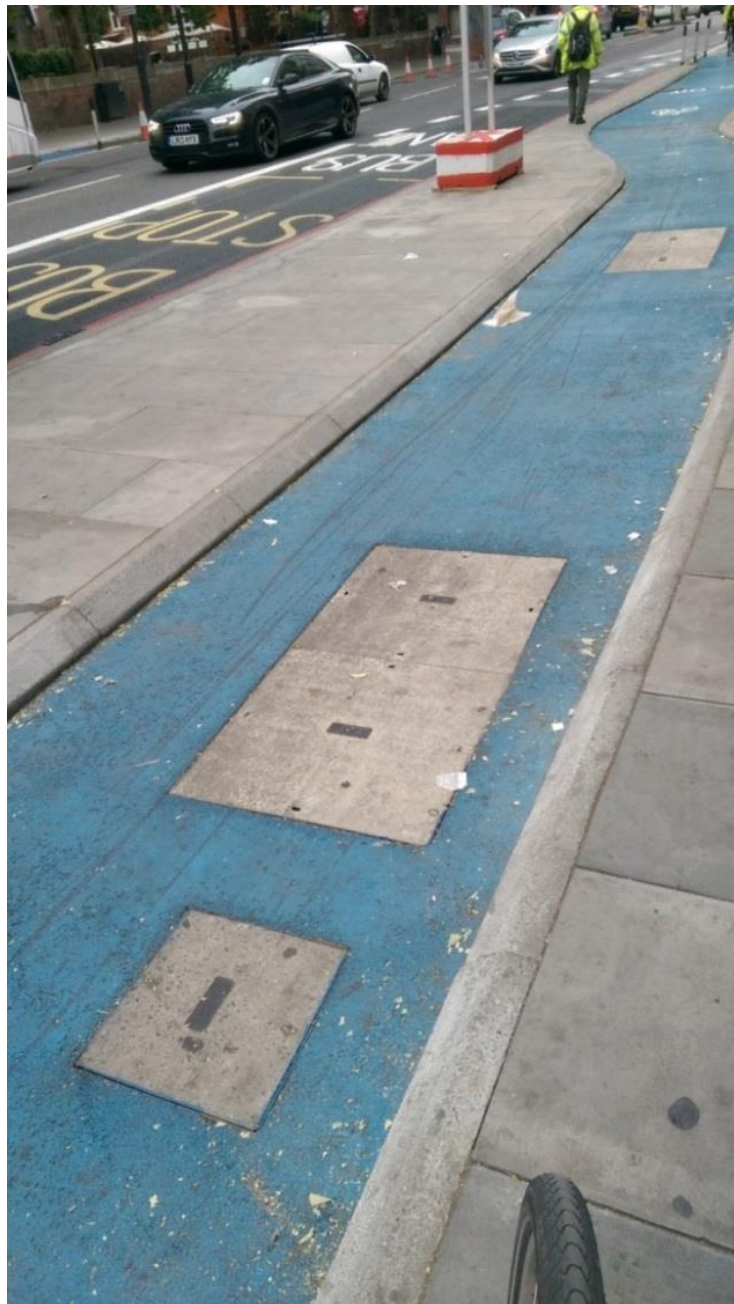
Bus stop bypass near Aldgate east station. Cycle skid marks can clearly be seen.
